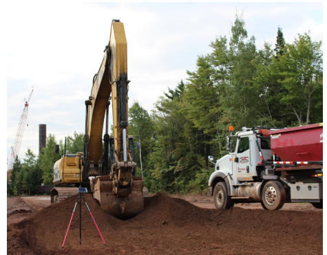
WE Energies - A.J. Mihm/F.D. Kuester Power Plants Marquette County, MI
